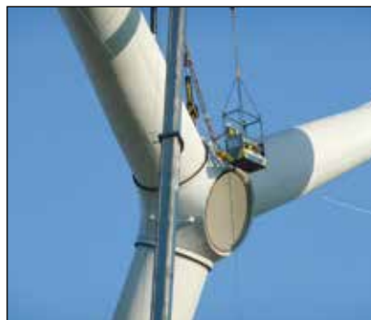
▼ The Enerpac SyncHoist system was used with one hydraulic cylinder to level and position the 95 ton, 115 m diameter rotor assembly of wind turbine.
