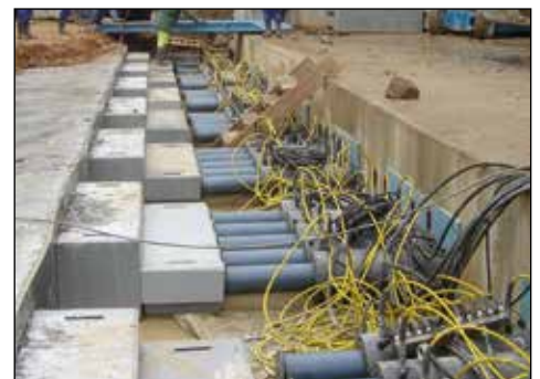
▲ Box jacking: Multi-point synchronous system to push hydraulically the tunnel segments under the railway.
