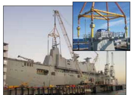
▼ An 4 x 110 ton SyncHoist system used to align steel blocks of the ship's control tower sections allowing gradual lift of the load and dynamic adjustment in relation to the centre of gravity during the lift.
